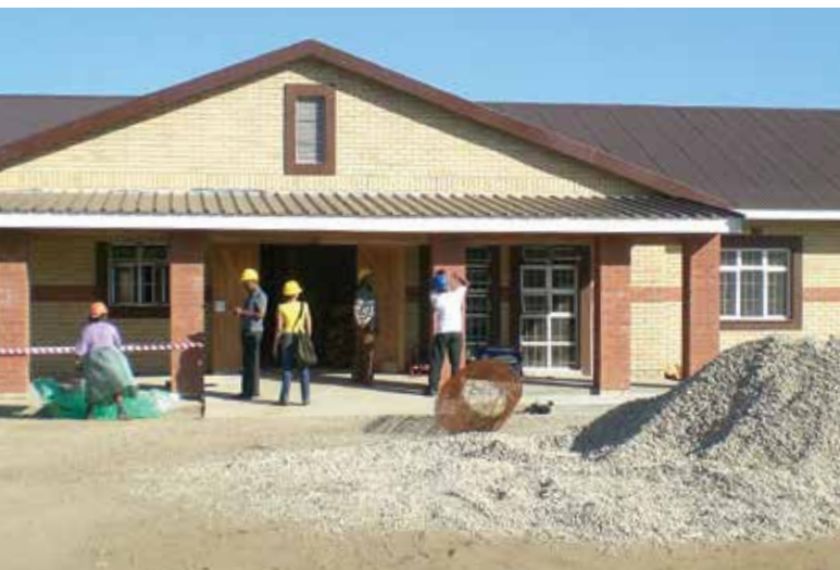
The KwaZulu-Natal community primary clinic under construction in 2007 in the township of Esikhawini, South Africa
